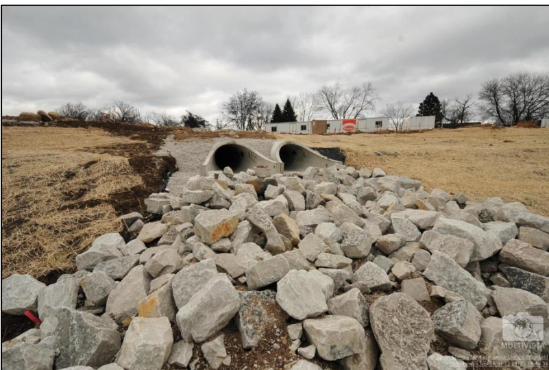
Figure 8 – Primary Storm Sewer
